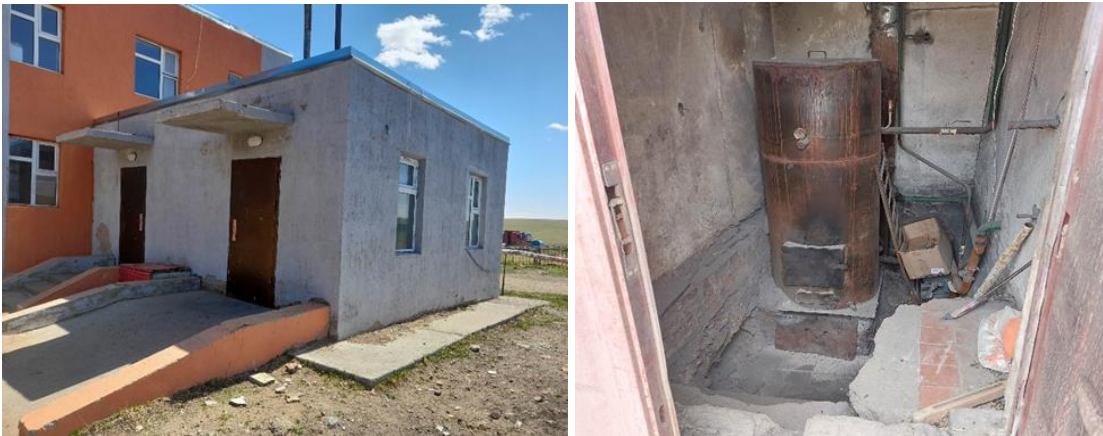
PICTURE 1. Heating boiler of the school, Dornod provinces’ Bayandun soum school
