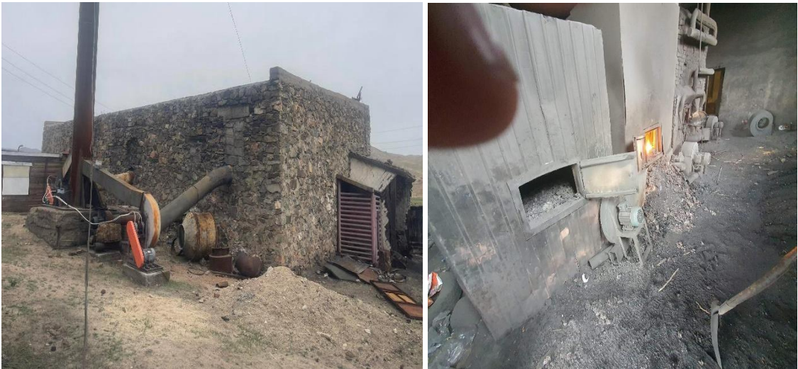
PICTURE 2. Heating boiler of the school in Khuvsgul province’s, Galt soum
