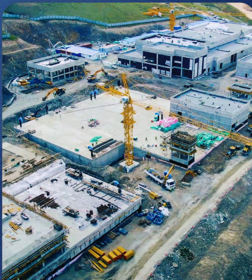
Water Purification Plant 2024
